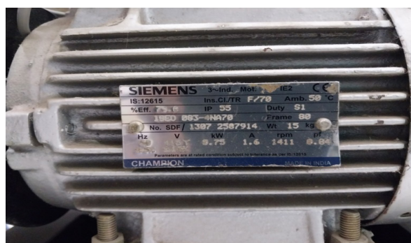
Fig. 6: Induction Motor name-plate specifications
