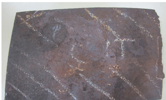
Figure 10: Corrosion under insulation on outside surface
