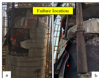
Figure 1: Tearing of urea reactor outer shell
