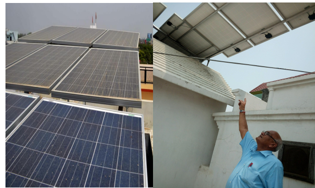
Fig.4: 5-Kw Roof Top Solar PV Plates Installed at Gomati Nagar, Lucknow
