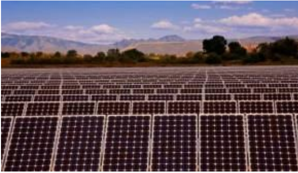
Fig.2: Solar Generation Unit
