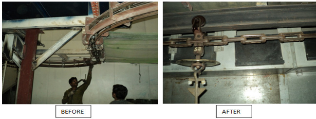
Chain conveyor section changed
